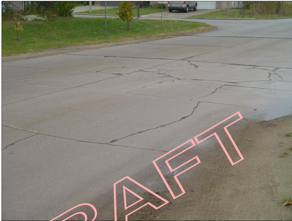
Photo 17 – Pulford Street - concrete distress about 20 m south of Northway Ave.
