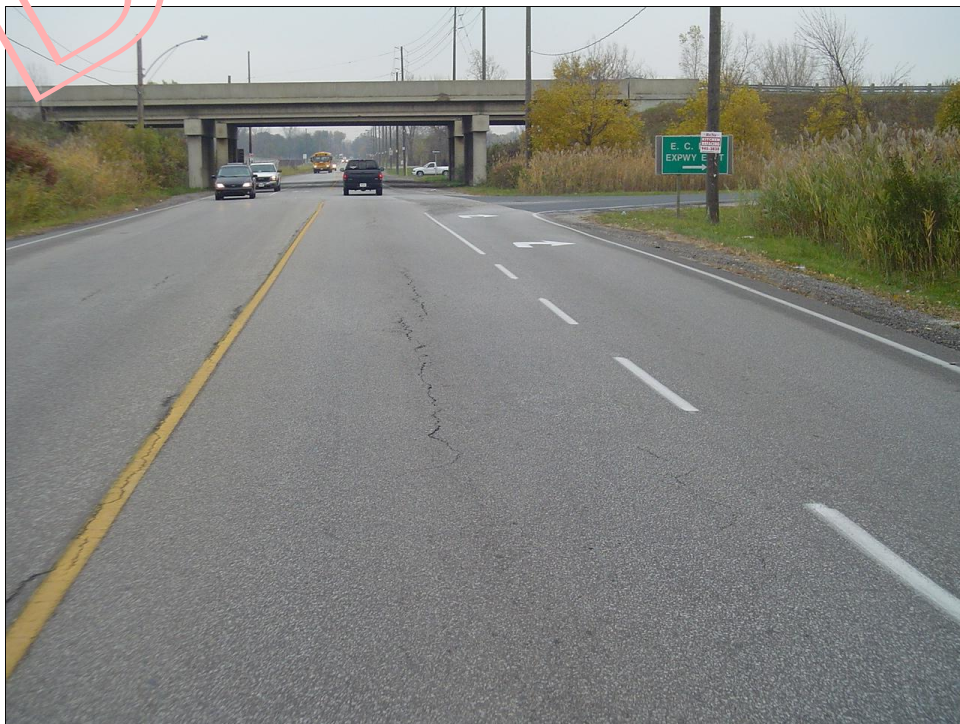
Photo 36 – Matchette Road – moderate longitudinal cracks
