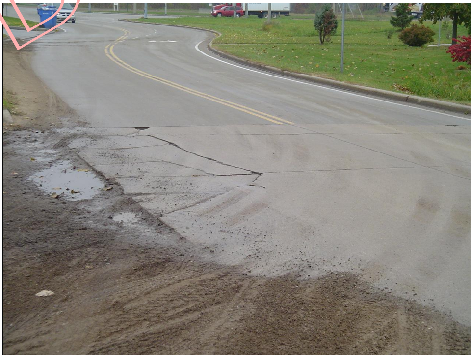
Photo 16 – Pulford Street – concrete distress about 50 m south of Northway Ave.
