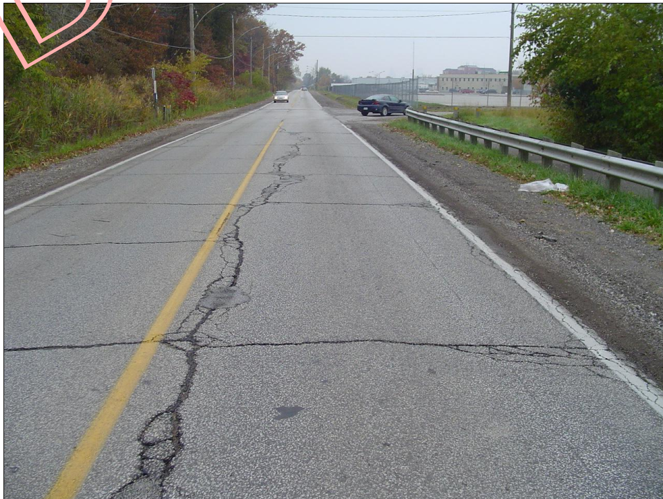
Photo 30 – Malden Road – very severe longitudinal/meander crack
