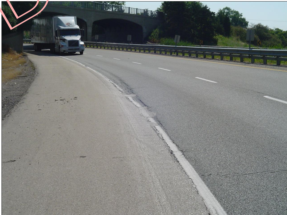
Photo 2 – Highway 401 westbound lanes just west of Talbot Road east. Note rutting and cracking at inner edge of pavement.
