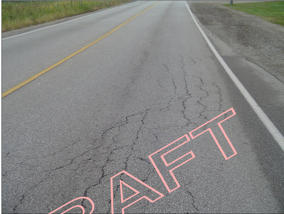
Photo 33 – Matchette Road – north of E.C. Row Expressway – alligator wheel path cracks
