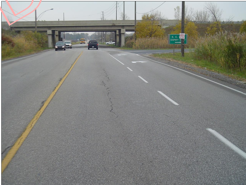
Photo 36 – Matchette Road – moderate longitudinal cracks
