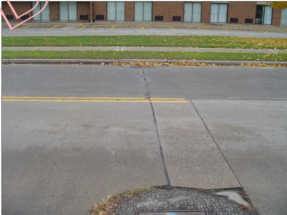
Photo 24 – Spring Garden Road – slight joint spalling
