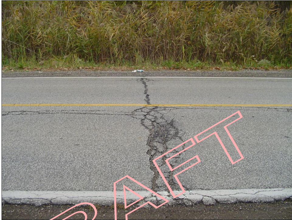
Photo 29 – Malden Road – very severe transverse crack
